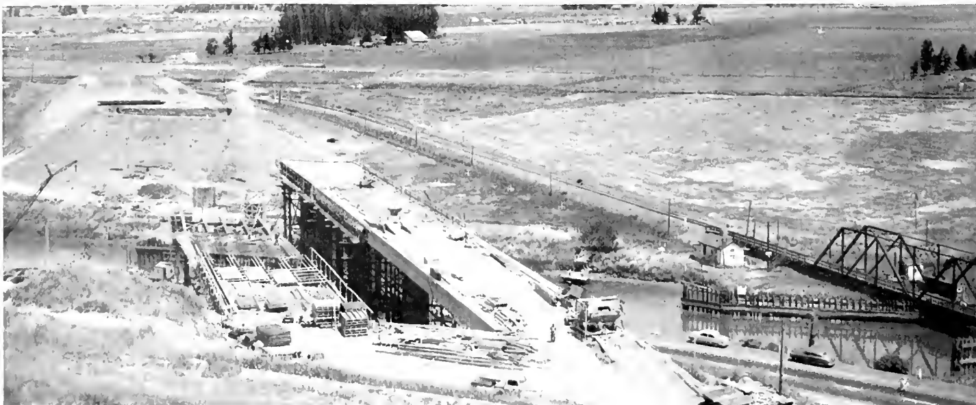
BELOW—Looking northeasterly at Petaluma Creek Bridge and Overhead during construction. North approach fill and abutment excavation on far side of creek. Northwestern Pacific Railroad Bridge at lower right.
